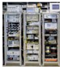
Optical loop test bed for investigation and development of S-, C-, L-band wavelength division multiplex systems with transmission rates up to 40 Gb/s per channel
